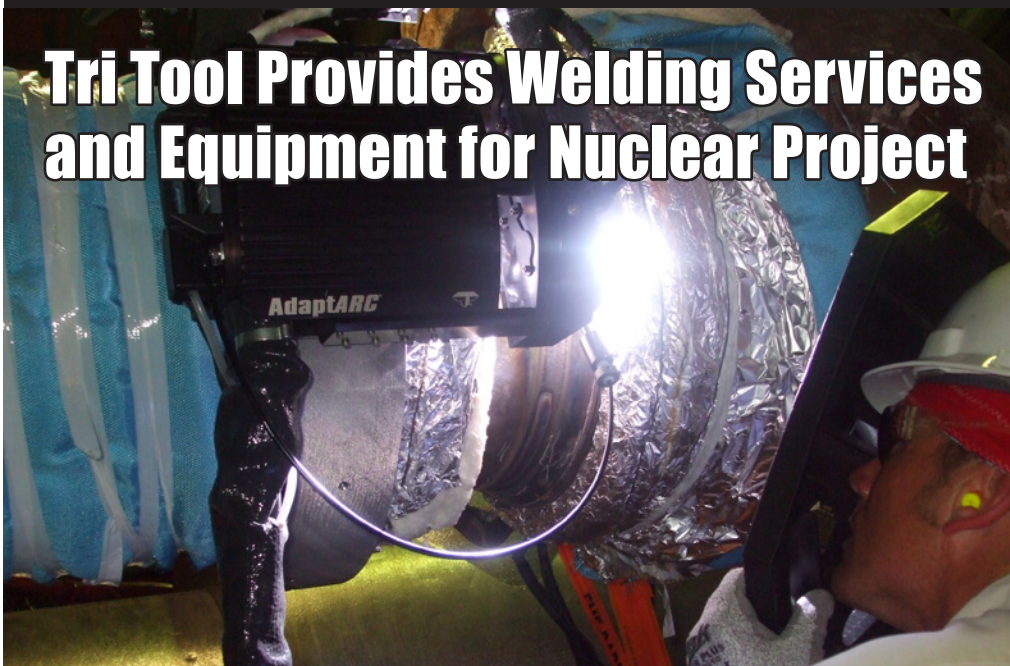
Above: The DualARC™ dual-process weld head is shown performing in-process weld on preheated 16" pipe. An oversized 20" mounting track was utilized to provide sufficient operational clearance for the weld head above the resistance heating pads.
